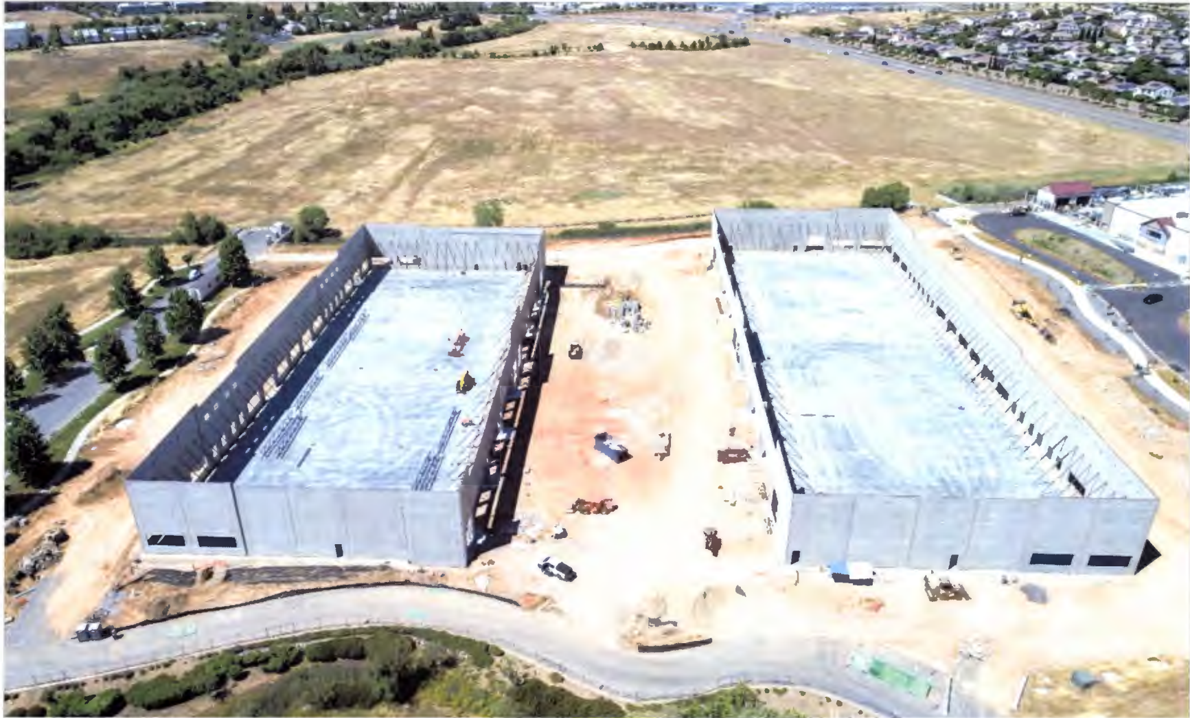
Construction of flex buildings (June 2024) looking north onto the GED site. Tractor Supply Company to the right, and the Carson Crossing Drive extension to the left.
