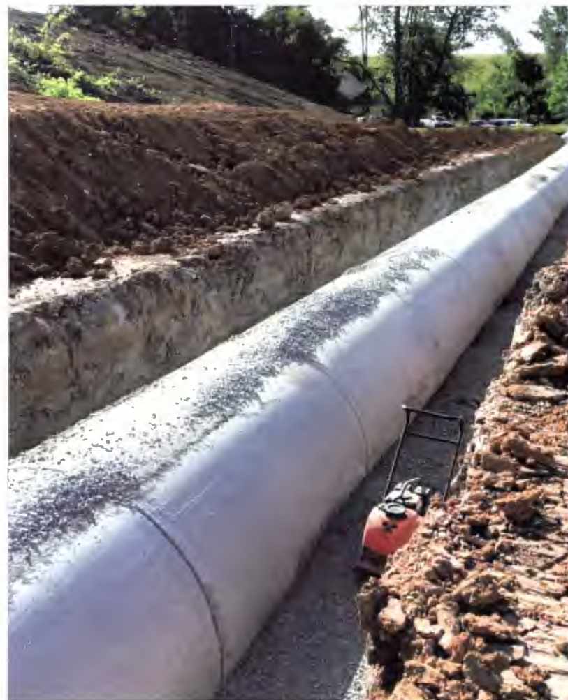
Concrete Drainage Pipeline
